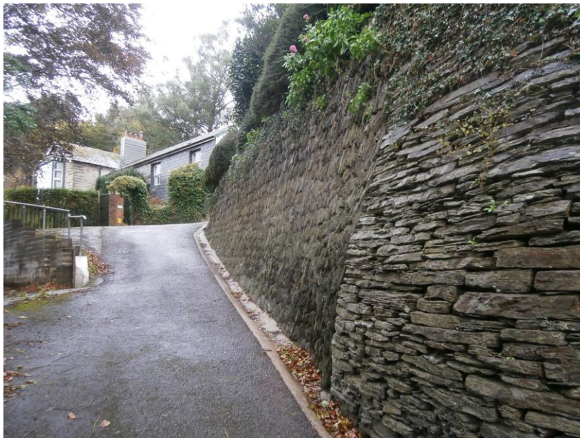
Looking uphill towards The Haven, the coursed stone lining the bank is a strong and attractive feature
